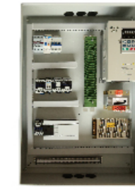
变频控制箱 Variable frequency control box
